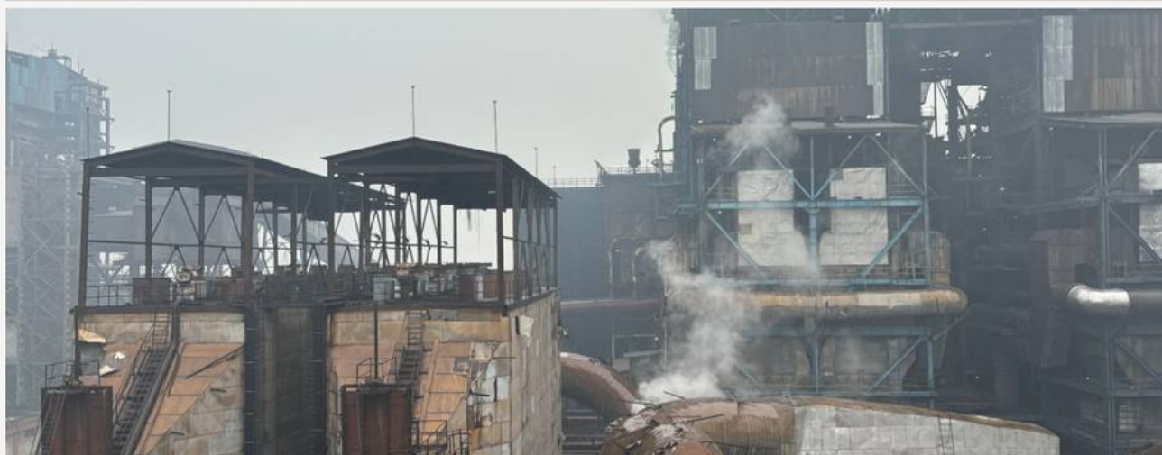
ESP INSTALLATION IN SERVICE
